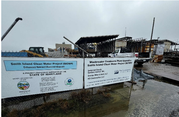
Construction of the new wastewater treatment facility taking place next to the aging facility
