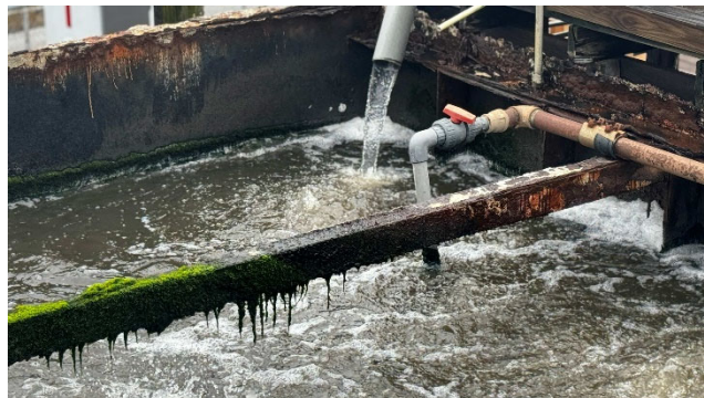
The aging wastewater treatment facility on Smith Island, severely corroded and in need of replacement
